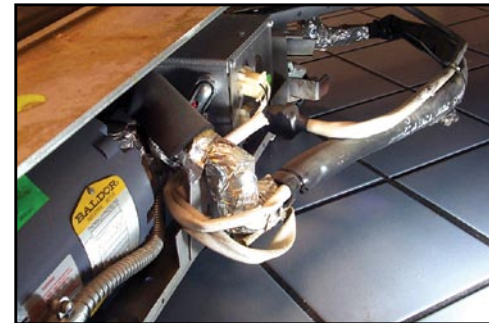
Heater tapes should be checked.
